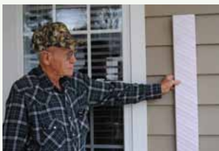
Mr. Green shows the reverse side of the insulated siding used on his home.
