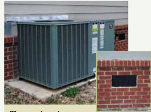
The outdoor heat pump unit was a major investment, but one that is quickly paying off, especially when combined with a brick foundation and vents
