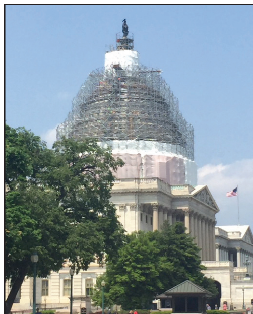
The U.S. Capitol is currently under renovation, which is scheduled for completion in time for Inauguration Day in January 2017.
