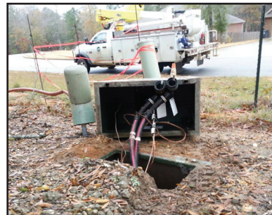
If you notice a damaged transformer, immediately contact CAEC at 1-800-545-5735.
