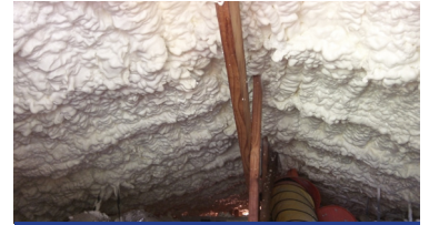
Boardwine says the foam insulation suggested has helped in lowering his energy bill.
